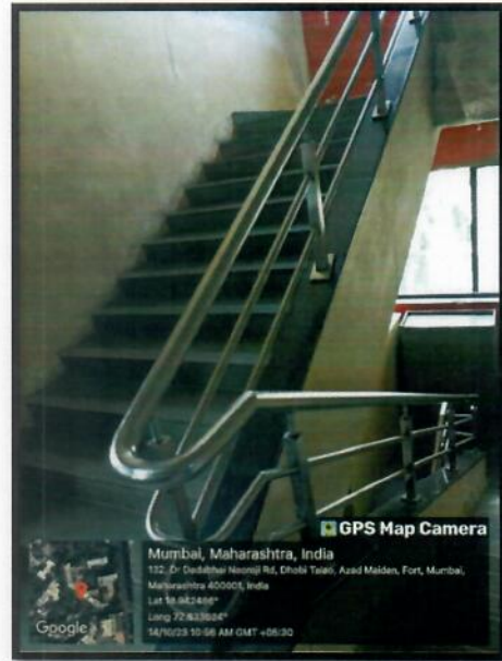
Railings alongside staircases for disable safety and access
