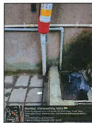
Waste Water In Seepage Tank
