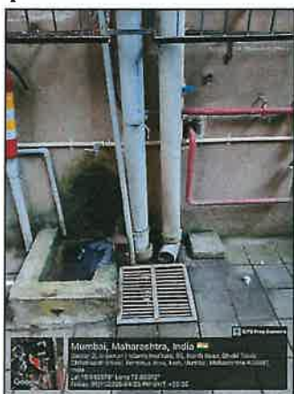
Disposal of waste water in seepage tanks
