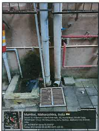
Disposal of wastewater in seepage tanks
